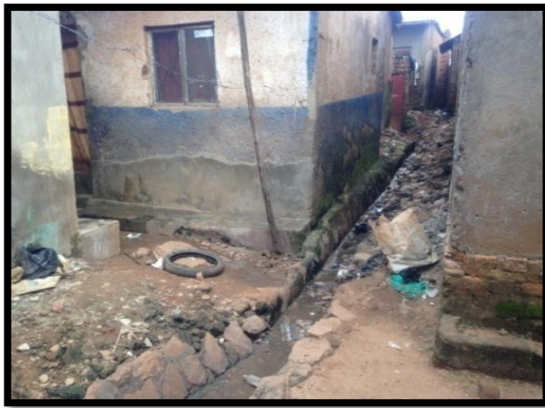
Drainage channel through houses which is dilapidated.
