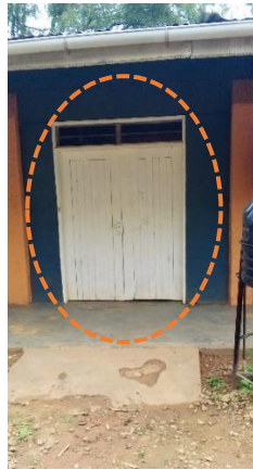
Figure 56: Opaque door at one of the dining hall
