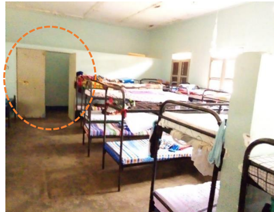
Figure 57: Opaque door in the girls dormitory towards the corridor leading to the toilet.
