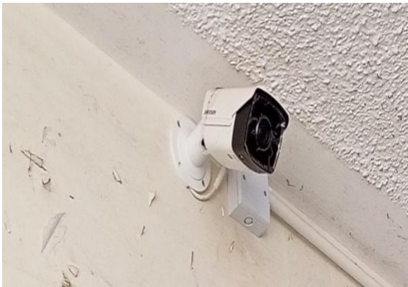
Figure 19: Showing an image of digital CCTV camera
