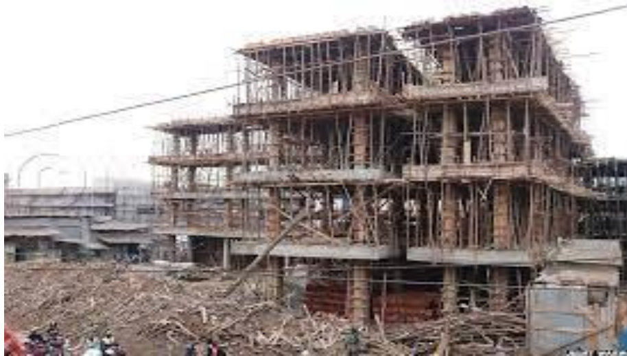
Figure 2-1: Collapsed Kisenyi Building
