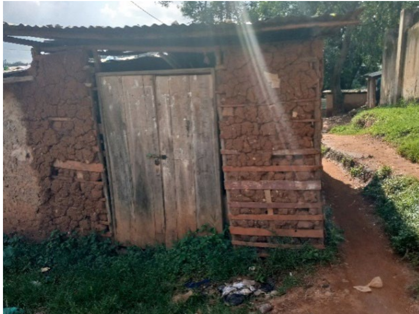
Figure 21:Disintegrating materials on some Informal Houses. (Source: Author)
