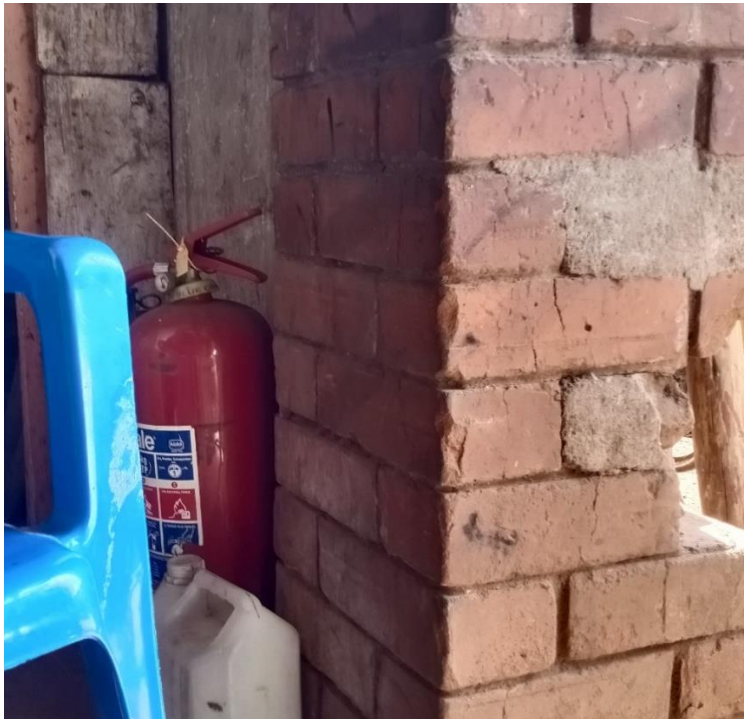
Figure 13: Fire extinguisher at Isa Auto garage
