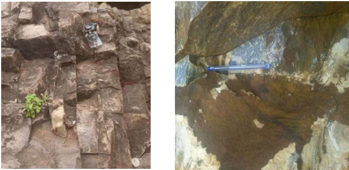
Figure 11: Shows both the major and minor joint sets in the mapped area
