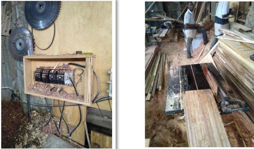
Figure 41: Electrical box(Left), attempts of electrical repairs by the workers(Right). Source: Author, 2021.
