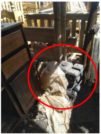
Figure 29: Generator in one of the workshops. Source: Author, 2021.
