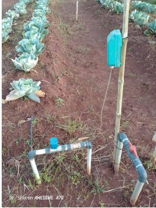
Figure 3.21: The Strega smart valve set up in the field.
