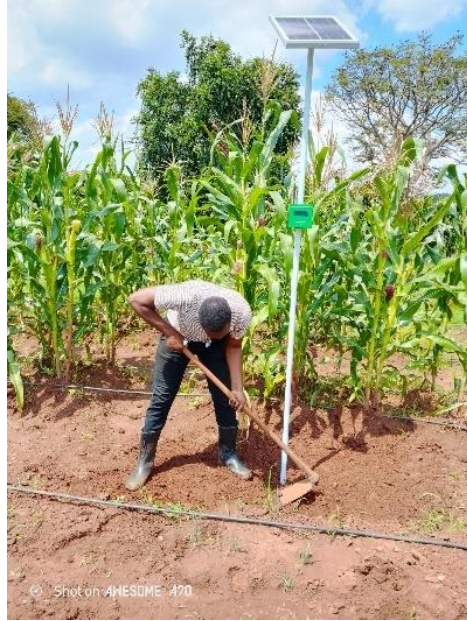
Figure 3.11: Back filling the dug pit having the erected 8ft tall steel pole
